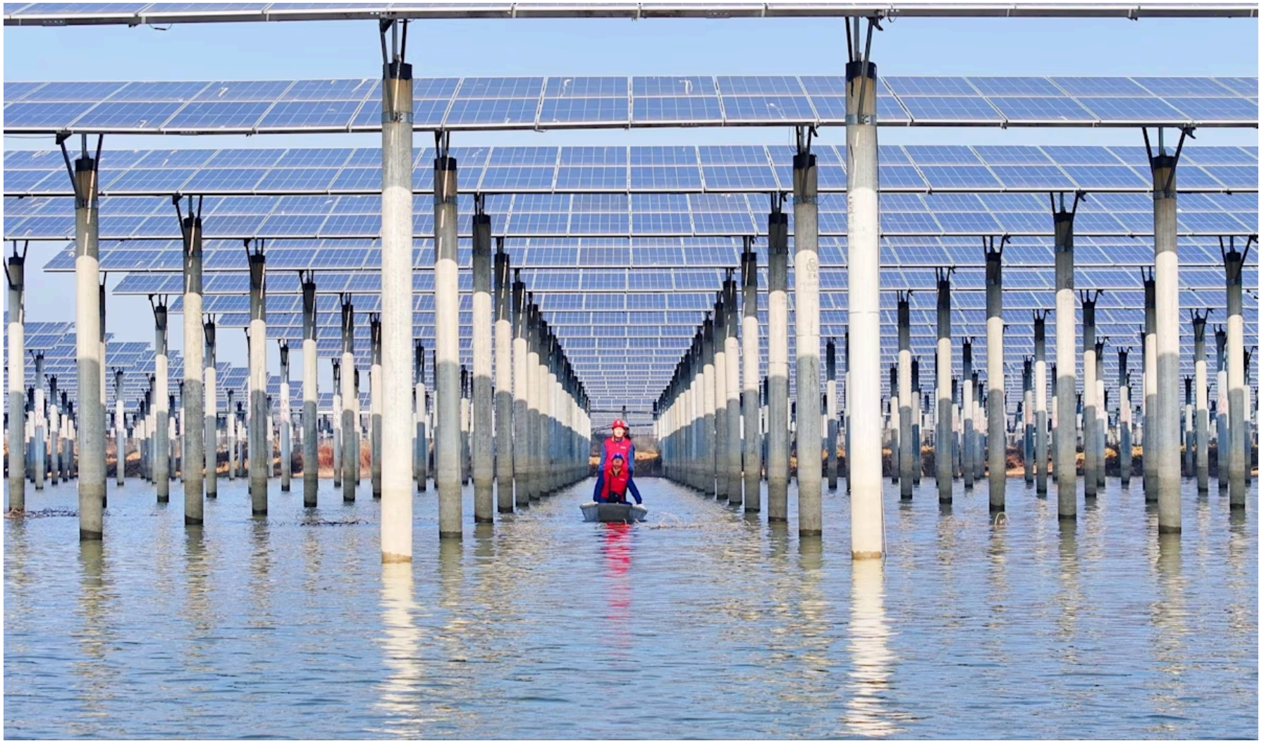
Inspectors check a photovoltaic power station in Tianchang, China. The country now controls more than 80 per cent of production for each key stage of solar panel manufacturing © CFOTO/NurPhoto/Reuters
